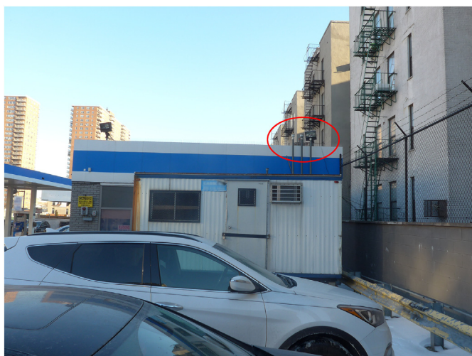
Fig. 1. The three vent pipes (enclosed by the red ellipse) on the right side of the convenience store of a gas station are <10 m away from the residential building. (For interpretation of the references to color in this figure legend, the reader is referred to the web version of this article.)
