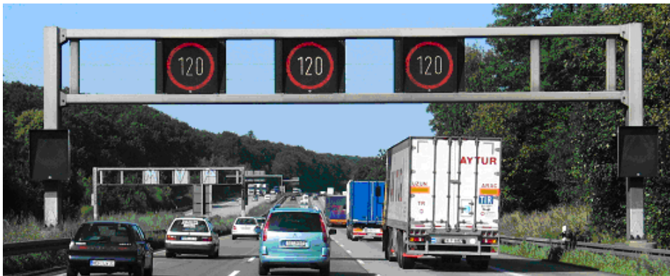
Figure 1: Dynamic Traffic Control System
