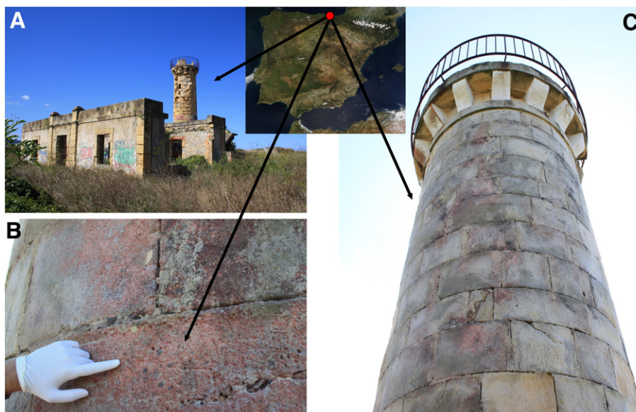
Fig. 1. (A) General view of La Galea Fortress, (B) red biofilm colonizing the sandstone from the Northside of the Fortress tower and (C) general view of the Northside of the tower showing the red biofilm on the sandstone blocks.
