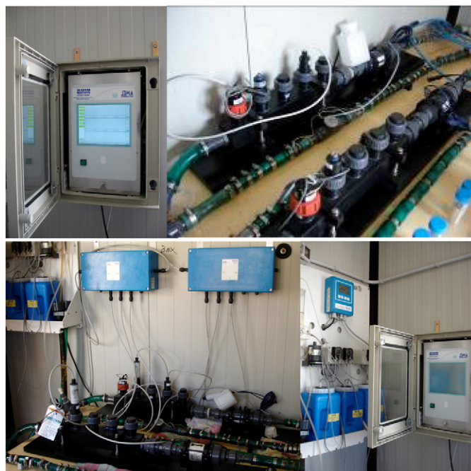
Fig. 1. Probes of the electrochemical integrated monitoring system installed in a power plant (BIOX probe in the frame).
