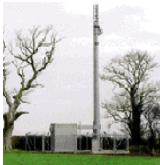
Fig. 1. RBS cabin and mast.
