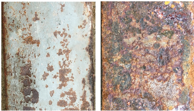
Fig. 2. Comparison of corrosion status of specimens.
