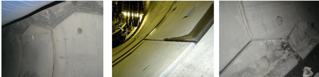
Fig. 1. Examples of concrete segment misalignments in different parts of tunnel lining.
