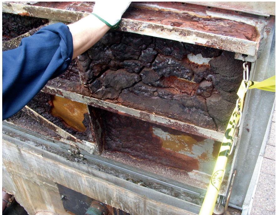
Traditional materials for manhole covers are subject to corrosion.
