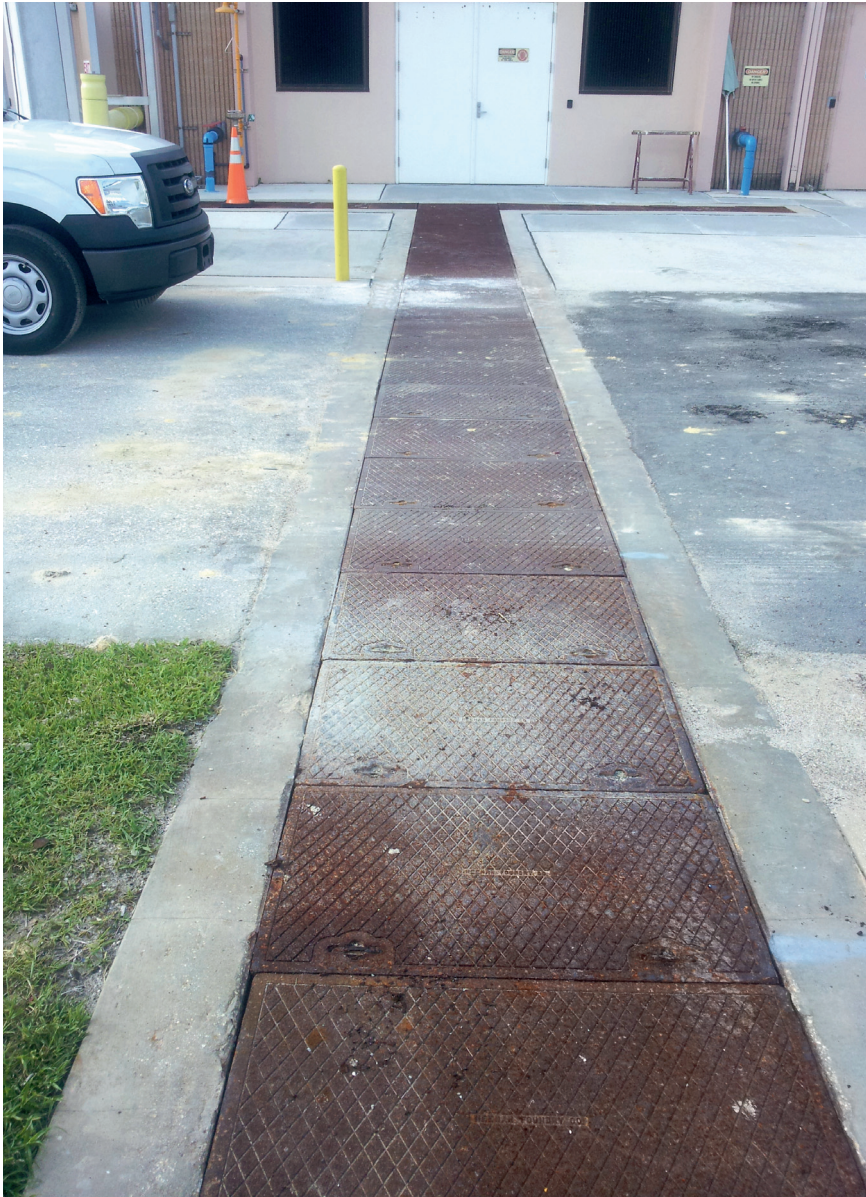
Corroded covers can be a problem in areas that need to stand up to heavy loads and severe impacts.
