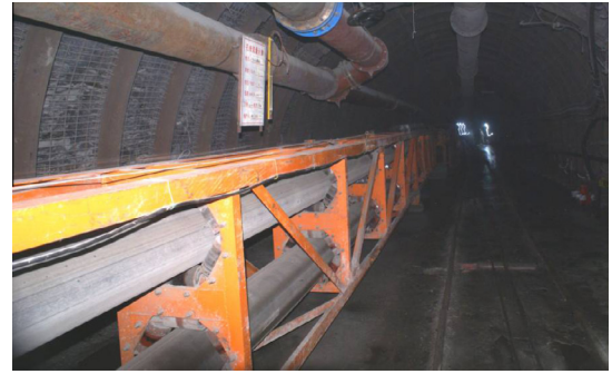
Fig. 2. Chinese first coal mine underground pipe belt conveyor.
