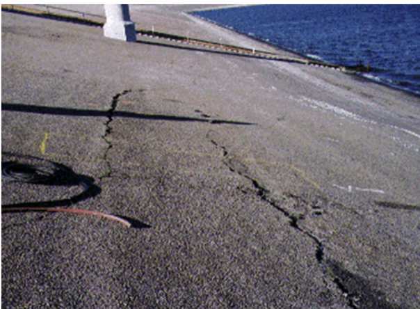
Fig. 1. Large cracks formed on the upstream side concrete of the Los Angeles Dam [9].
