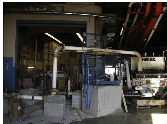
Fig. 1. Pump, beginning and end of the pumping circuit. Concrete flows from the pump in the pipes (bottom right) towards the left (in background). The final stretch of the circuit is elevated to allow the concrete to be pumped back into the reservoir, or take a sample.
