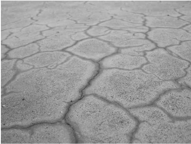
Fig. 1. Early age shrinkage cracks in a concrete slab on grade.
