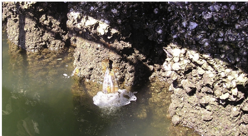
Fig. 2. Perforation and ground water draining into harbour waters at extreme low tide, showing perforation of a U profile pile near the junction between the web and the flange of the pile (Newcastle Harbour).
