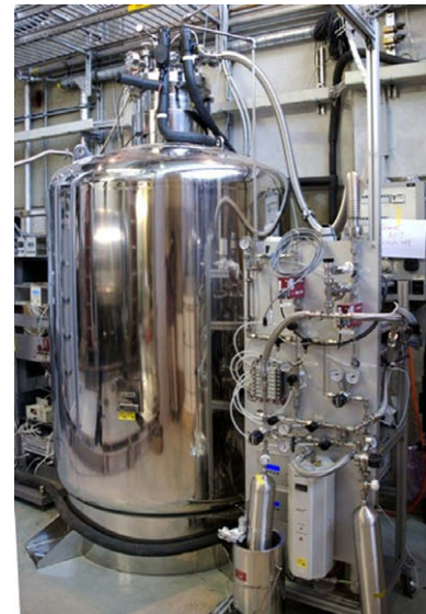
Fig. 3. LXe cryogenic tank with gas purification system.
