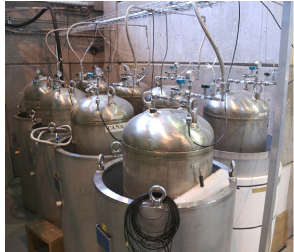
Fig. 2. GXe storage tank.
