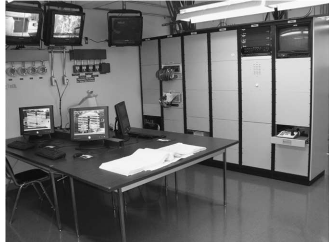
Fig. 3. Interconnect room. The interconnect room located within the test building at SMiRF is used for checkout of the control and data systems for SMiRF and CCL-7.
