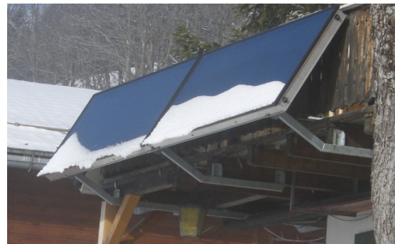
Fig. 2: Balustrade mounted collectors damaged by snow load
