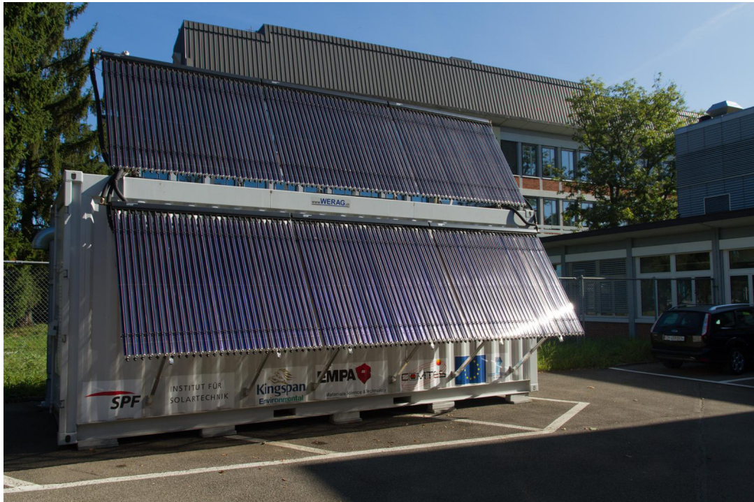
Fig. 1. Picture of the complete system from the outside. Solar collectors with an active area of 18 \text{ m}^2 are mounted on top and on the side of the shipping container.
