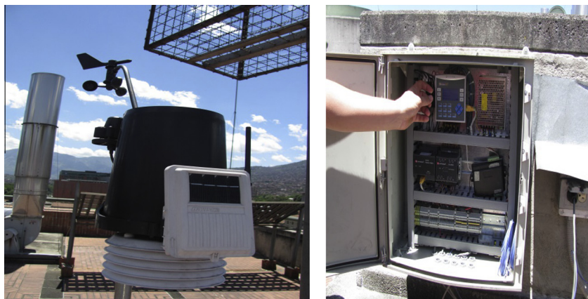
Fig. 1. Equipment used for monitoring the solar modules. Left. weather station. Right. PLC.
