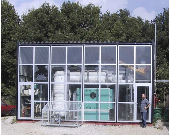
Fig. 1. Picture of the Viking gasifier in operation.
