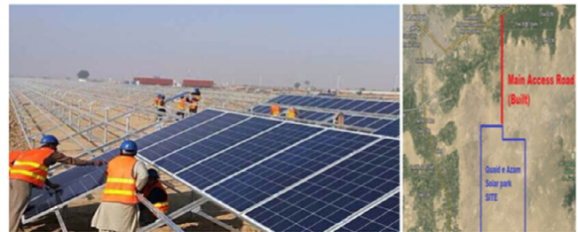
Fig. 5. Pakistan 1st 100 MW solar power plant (Chinese company) 2015 (Tso and Yau, 2007).
