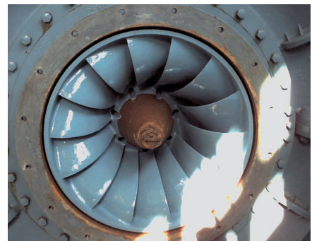
Figure 5. Application of Belzona 1341 (Supermetalglide) ® in progress to runner. This coating has been proven to reduce surface friction, resulting in higher operating efficiency in fluid flow equipment such as turbines and pumps.
