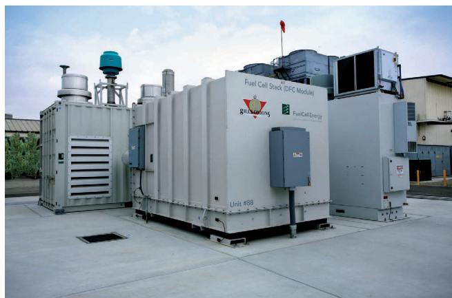
Gills Onions in Oxnard, California, has been operating at 600kw molten carbonate fuel cell system supplied by FuelCell Energy since 2009. It runs on biogas from the fermented onion juice. Photo credit: FuelCell Energy.
