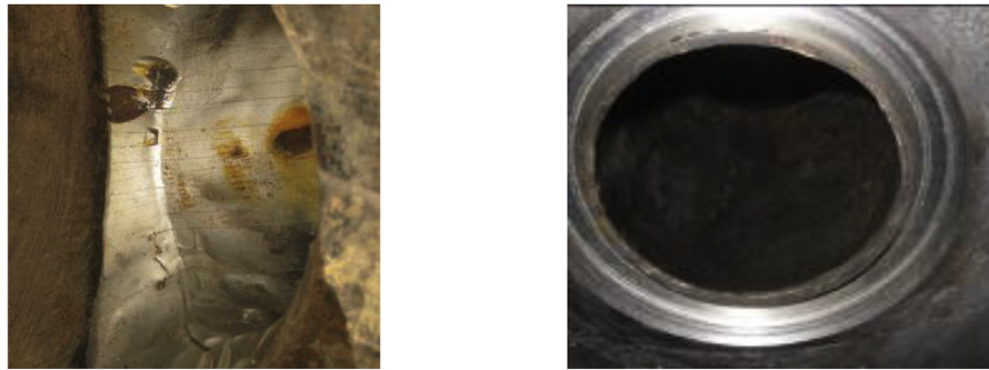
(a) Multifunctional four-way bypass entrance (b) Multifunctional four-way bypass outlet
