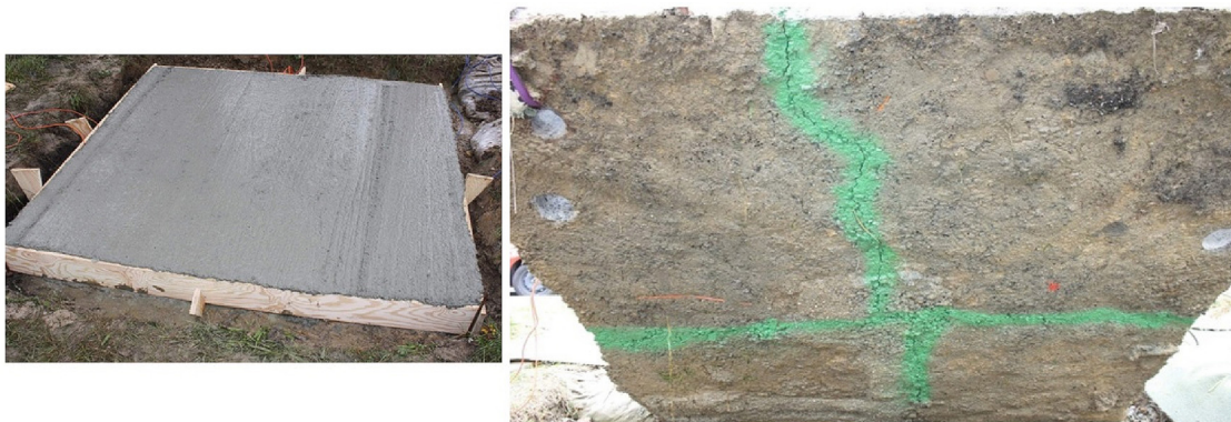
Figure 1 Casting of the steel-fibre reinforced concrete slab and cracks at the lower surface of the failed steel-fibre reinforced concrete slab after its lifting up.
