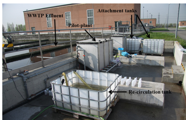
Fig. 1. Structure of the pilot-plant located at the Milano-Nosedo WWTP.
