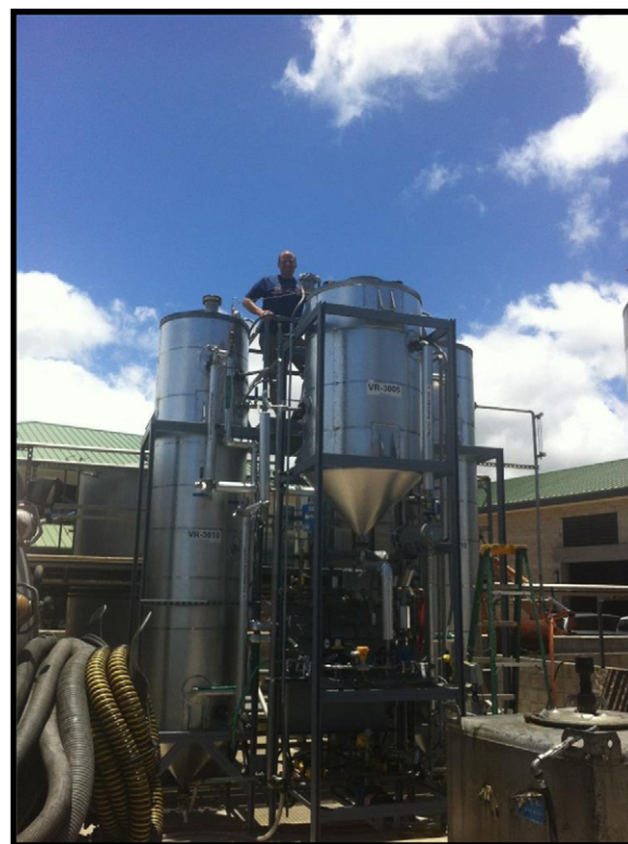
Fig. 2. Installed pilot scale HRAD system.
