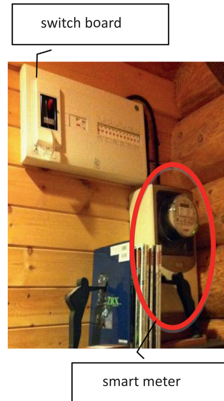
Fig. 1. Picture of a smart meter installed in a household.
