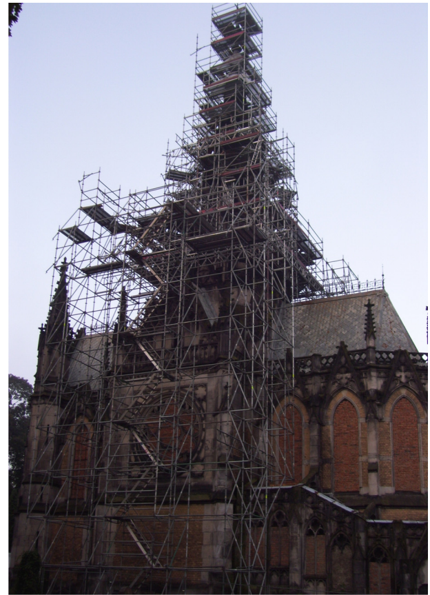
Fig. 2 – Unanchored scaffolding at Scheibler Chapel in Lodz (Poland).
