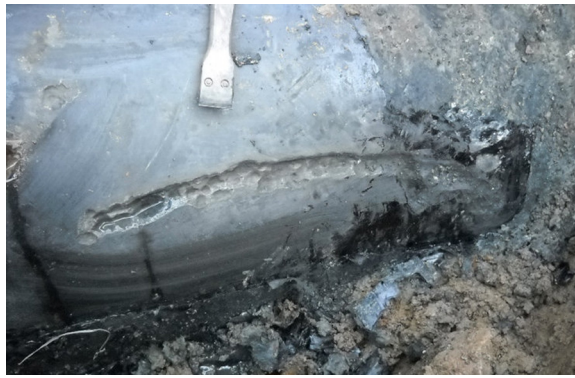
Fig. 2. Zoom on the defect site.
