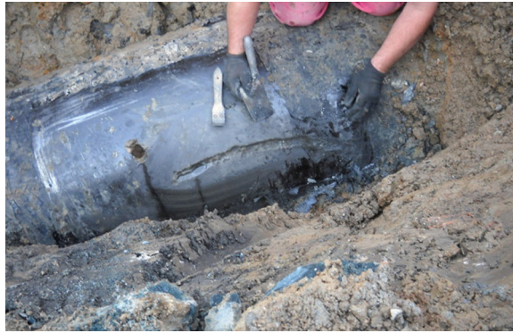
Fig. 1. View of pipeline corrosion failure.
