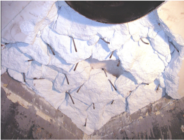
Fig. 1. The part of the combustion zone structure in the heating unit used in oil refineries damaged by explosive spalling (metal anchors can be seen on the photograph).
