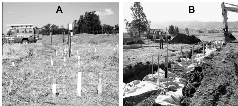
Fig. 1. (A) Pilot-scale PRB with piezometers and monitoring wells in ASS terrain on Shoalhaven Floodplain, southeast NSW and (B) installation of the PRB.
