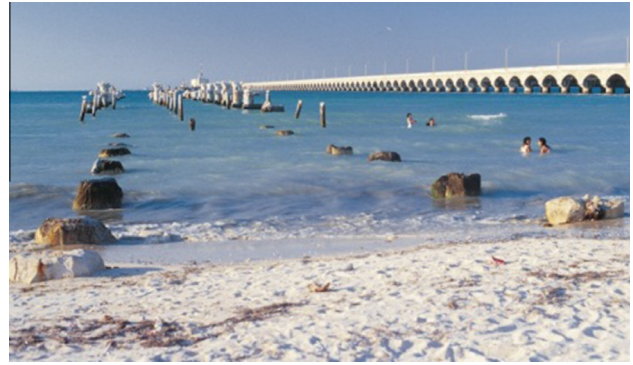
Fig. 1. Progreso Pier, Mexico – the pier in the background was constructed in 1940 and used stainless steel reinforcing bar whereas the pier in the foreground was constructed in 1969 and used carbon steel reinforcing bar (Courtesy of the Nickel Institute).
