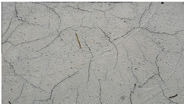
Fig. 2. Shrinkage in slab due to inadequate moist curing in severe hot weather conditions.
