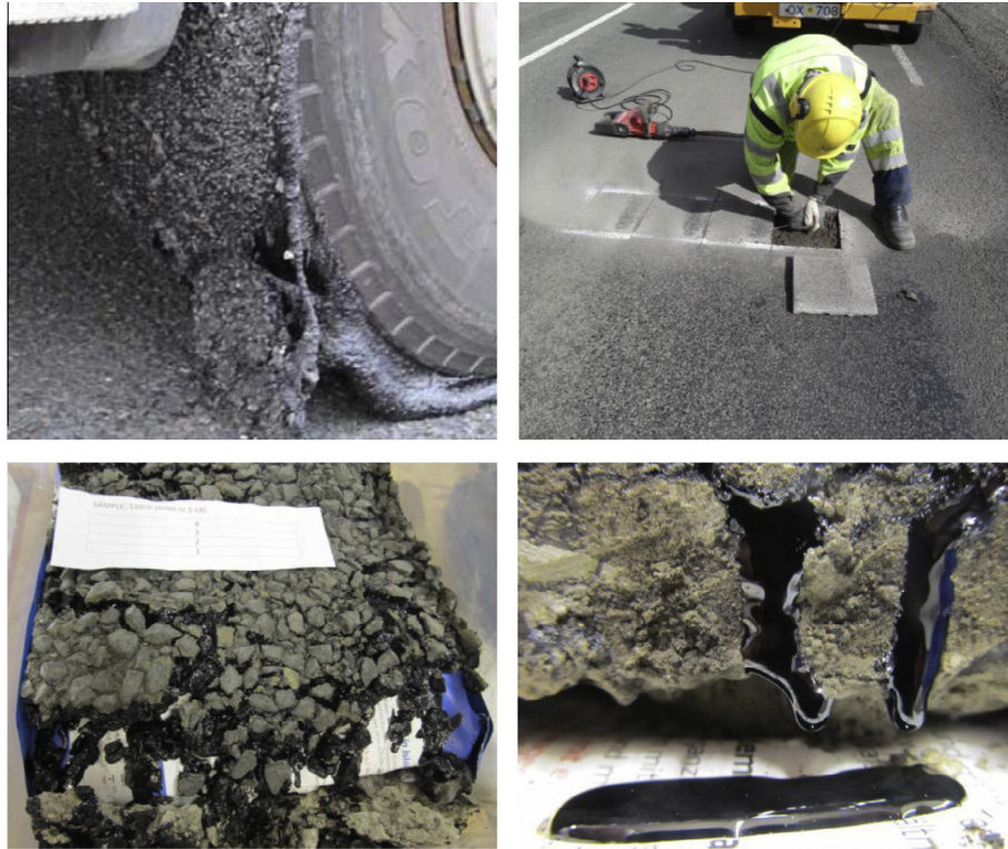
Fig. 1. Extensive surface dressing damage.
