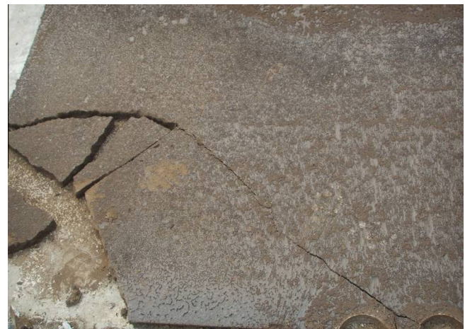
Fig. 2. After lifting the track slab above, foam layer on the surface of hardened CAM was seen. Foam layer would decrease the bonding strength between CAM filling layer and track slab seriously.
