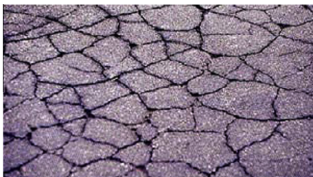
Fig. 1. Fatigue cracks in asphalt pavement.
