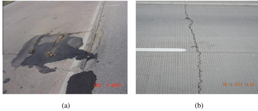
Fig. 1. Major CRCP distresses: (a) punchout; (b) spalling.
