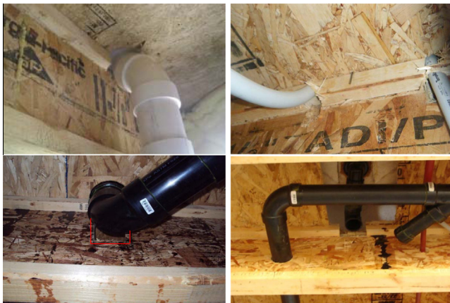
Fig. 1. Flange notch at construction site.
