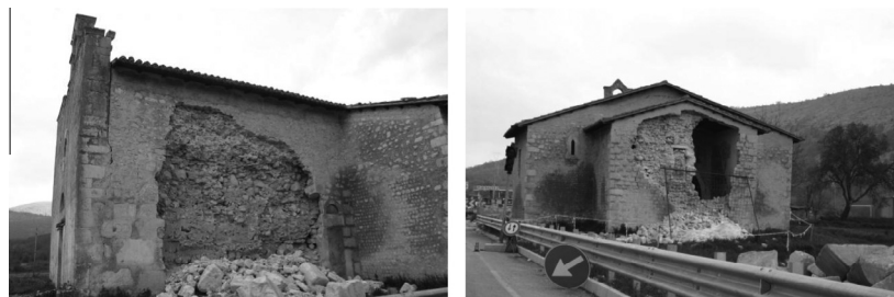
Fig. 1. Out-of-plane failure of stone masonry walls without transversal connections due to horizontal seismic actions, L'Aquila, Abruzzo, Italy.
