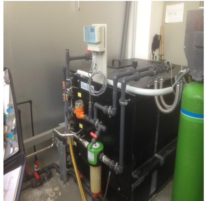
Fig. 2. Soft water tank, black. The concentrated caustic soda was pumped backwards into the soft water tank and accumulated there to form a highly concentrated solution.
