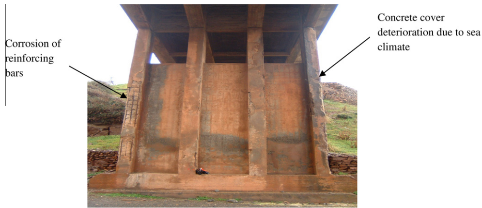
Fig. 2. A view of pile degradations.
