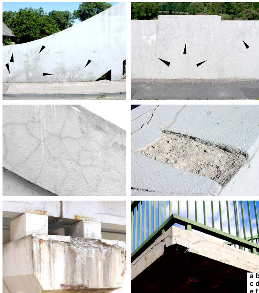
Fig. 1. In situ observation of ASR. (a), (b) cracks through the face-side (indicated by black arrows), (c) detailed view of the net of cracks, (d) detailed view of the spandrel panel over the pillar, (e) front of the pillar damaged by concrete spalling, (f) cracks through the landing front.
