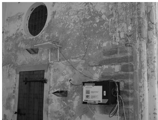
Fig. 2. South wall of the choir showing serious damage.
