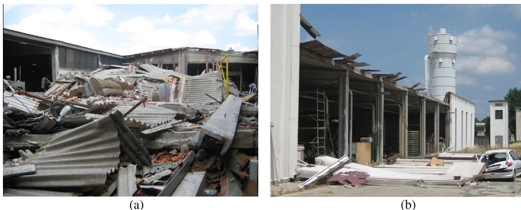
Fig. 1. (a) Collapse of a precast RC building, and (b) collapse of precast vertical panels due to the earthquakes in the Emilia Romagna region.
