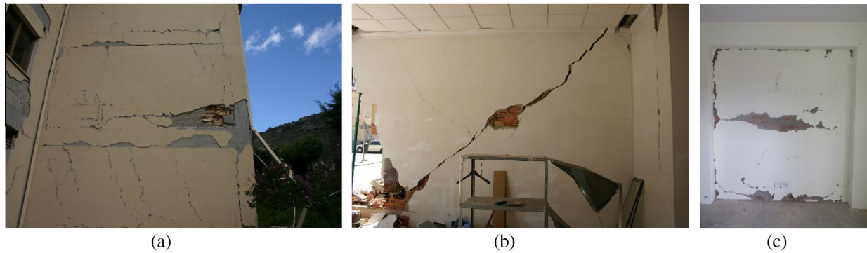
Fig. 1. Typical damage observed on in-plane IM walls: (a) detachment of the surrounding RC frame in the L'Aquila (Italy) earthquake, (b) diagonal cracking in Lorca (Spain) and (c) in the Nepal earthquake.
