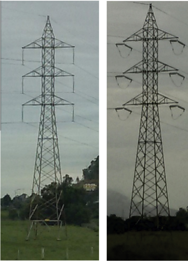
Fig. 1. Transmission line towers with staggered bracing: suspension (left) and angle (right) towers.
