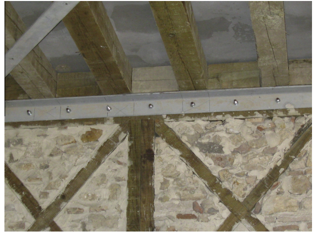
Fig. 1. Connection between a new timber floor and timber-framed masonry walls using steel angles.
