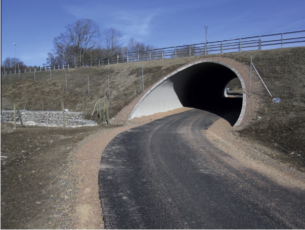
Fig. 1. A typical corrugated flexible culvert under the E6 road at Saltkällan, Sweden.
