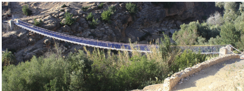
Fig. 1. Polyester-rope suspended footbridge (Ait Bayoud, Morocco, 2013) showing hand and under-deck ropes, as well as two short towers.
