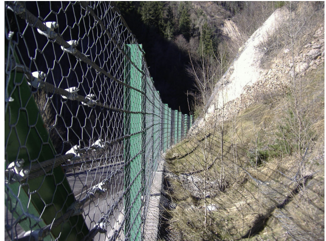
Fig. 1. A typical semi-rigid rockfall protection barrier installed in the Autonomous Province of Bolzano (Italy).
